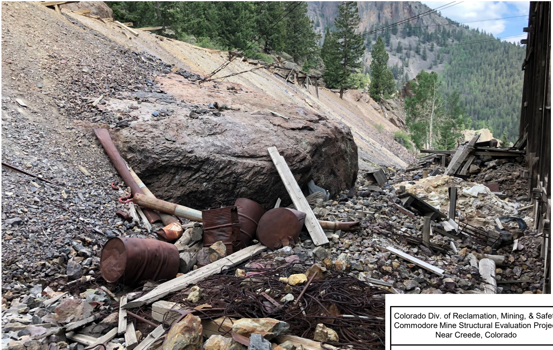
West side of Ore Sorting house and covered trestle showing accumulations of waste rock and debris. Note rock outcrop at center. View due south on June 23, 2021.
