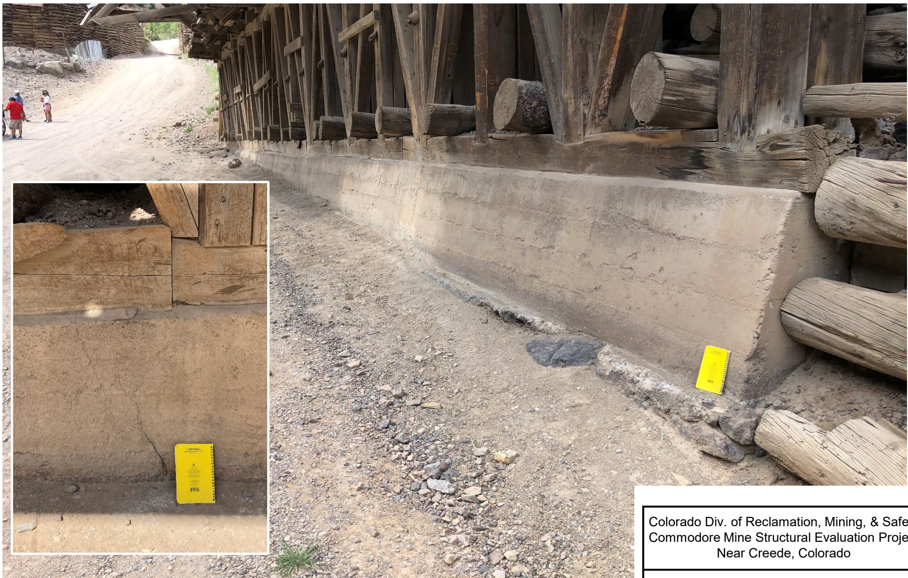
Concrete footing along west side of Ore Sorting House. View due north on June 23, 2021. Inset shows typical crack in footing.
