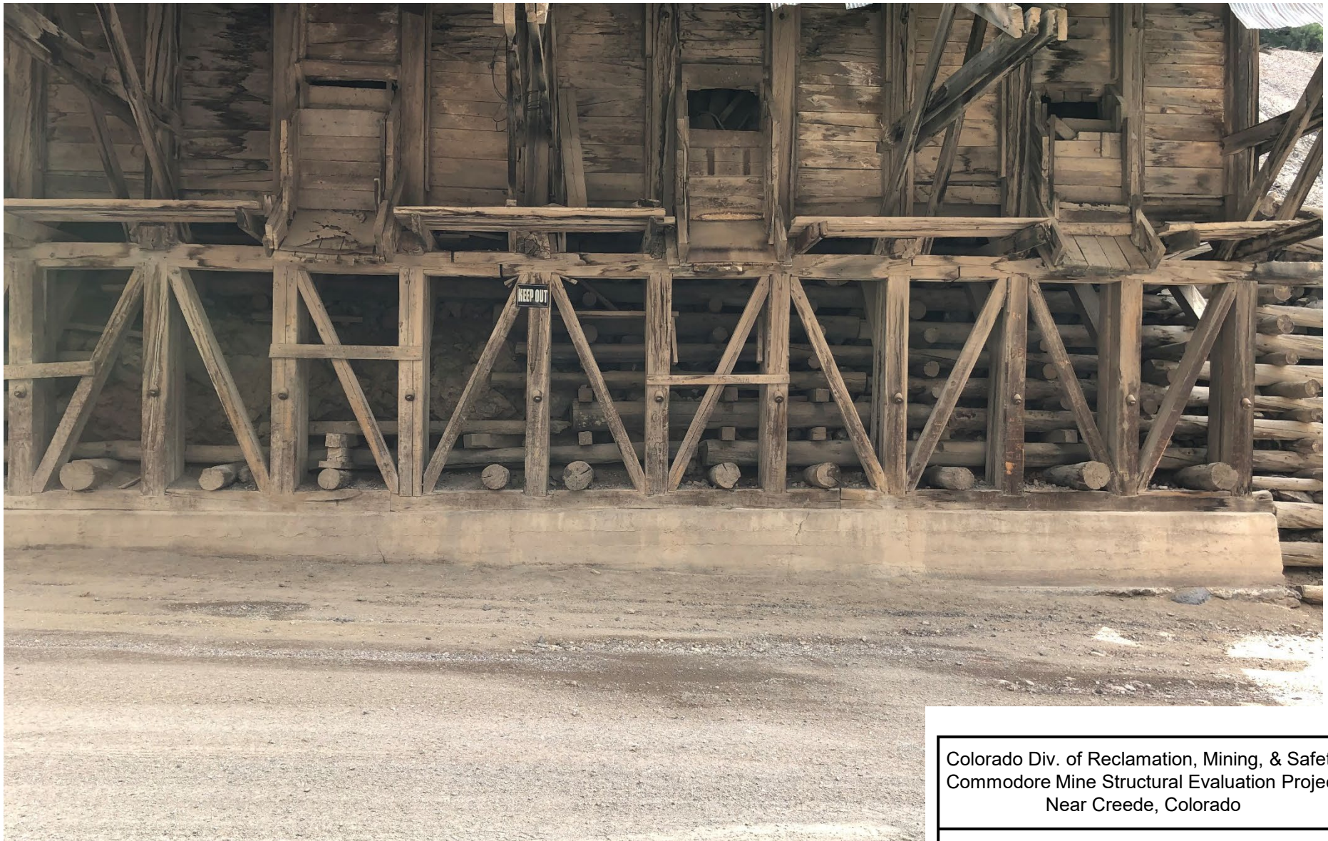
Cribbing behind west façade of Ore Sorting House. Note potential bedrock exposure and gap in cribbing at left. View due east on June 25, 2021.
